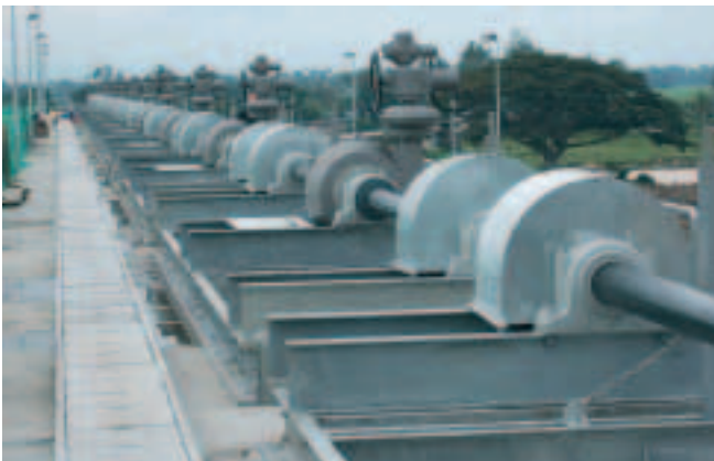
For an irrigation project in Malaysia large multi-turn GS gearboxes without end stops are used. The illustrated plant shows how the position of the weir penstock is controlled.
